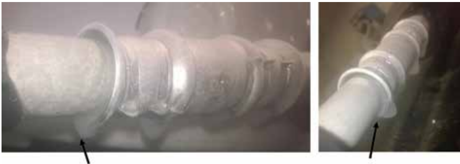
Ice formation between the tube and the fitting during the freezing cycle
